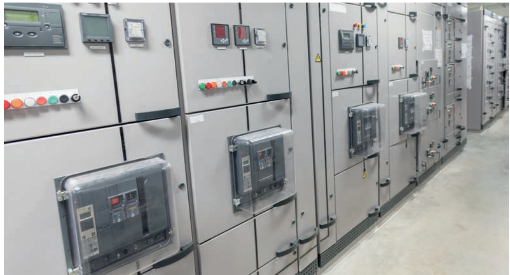
Figure 4.1 Switchgear in a distribution substation
